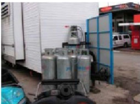
Secured to other cylinders
