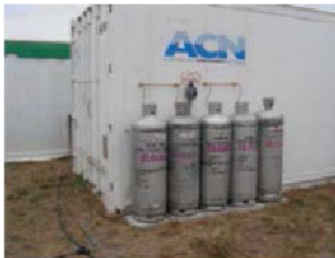
Secured and on a stable base
